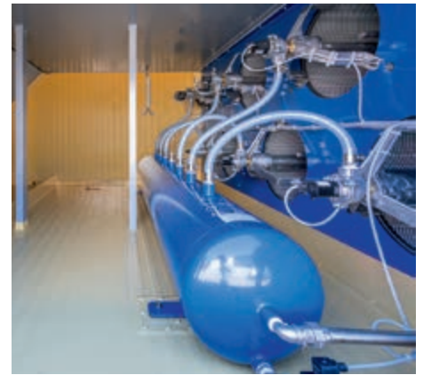
Filter cleaning with compressed air
