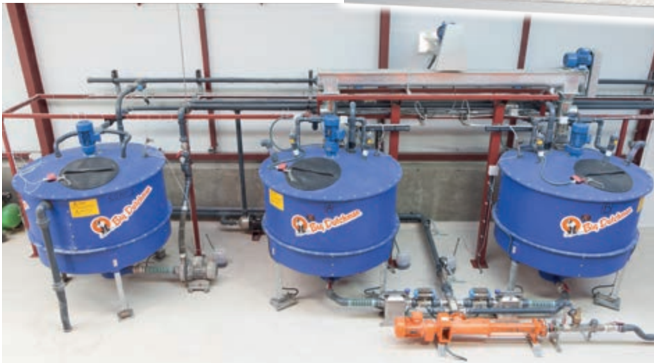
Feed kitchen: 2-tank system with rinse water tank
