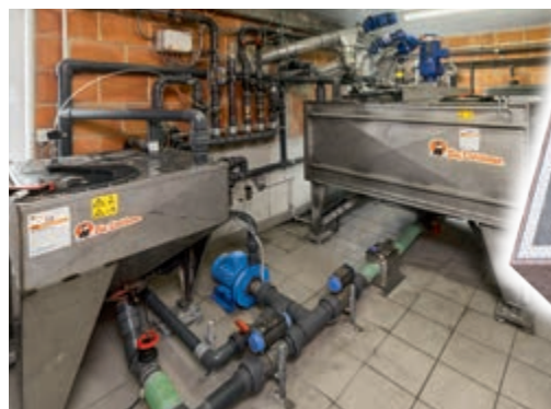
Feed kitchen: 1-tank system with weighed rinse water tank
