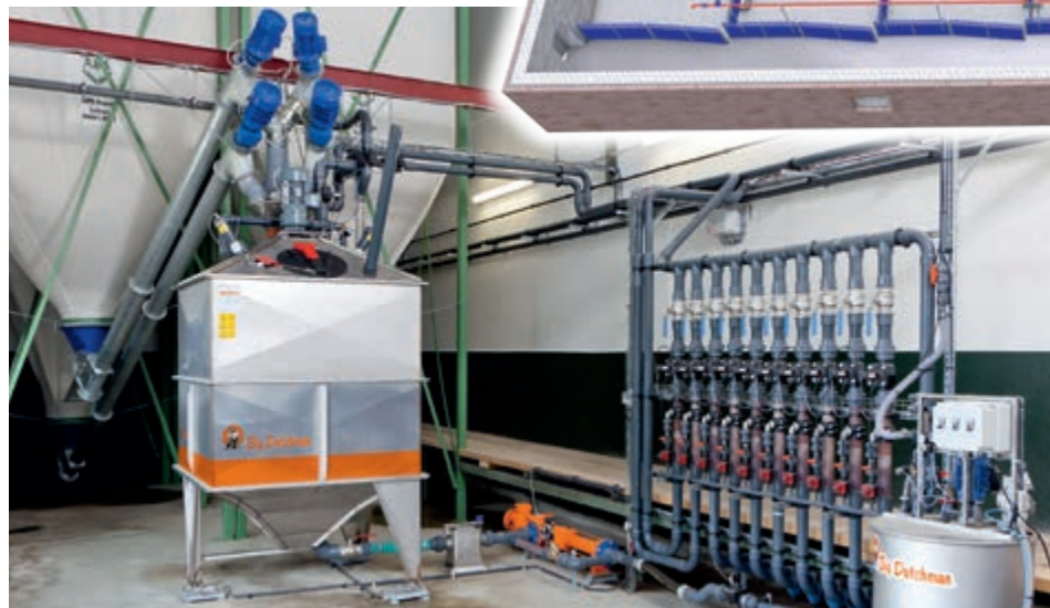
Feed kitchen: 1-tank system with filled branch lines for a finishing house with 2000 pigs
