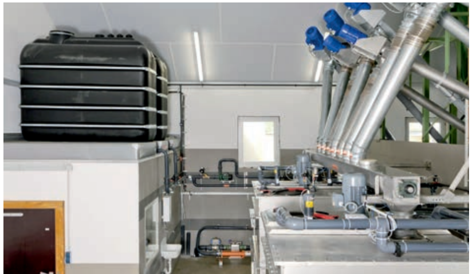
Feed kitchen with 2-tank residue-free feeding system and two 2000 L fresh water tanks
