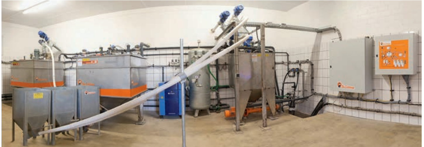
View into a feed kitchen with a HydroMix liquid feeding system for piglet rearing based on compressed air and a 1-tank, residue-free system for sow feeding
