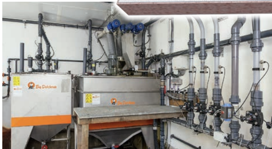
Feed kitchen: 1-tank system with rinse water tank and four JET branch lines
