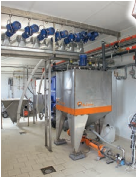
Feed kitchen: 1-tank system (residue-free) with compressed air
