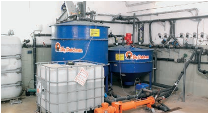
Feed kitchen: 1-tank system with weighed rinse water tank
