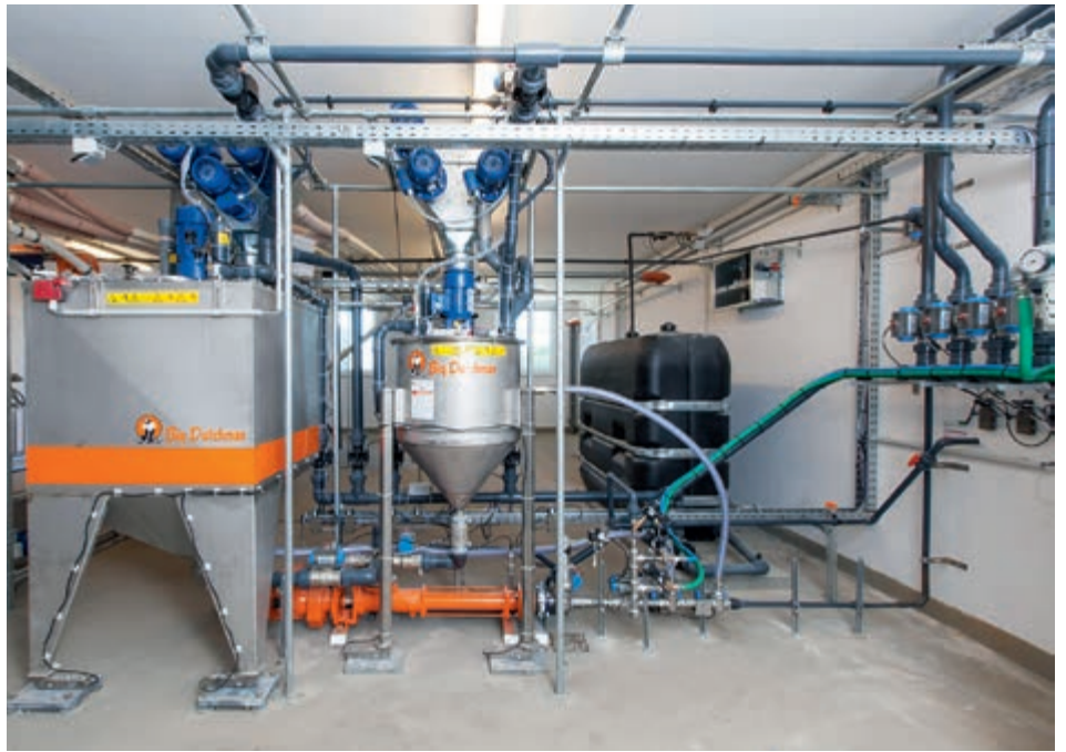
Feed kitchen: 2-tank system with rinse water tank
