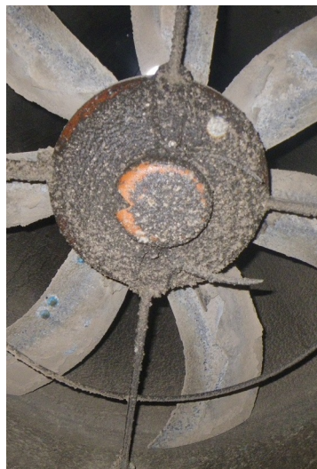
Figure 2: Fan with guard cap after 7 months of operation
